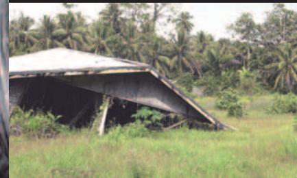
Rare damage scene. Few post-tsunami photos of Arop remain because the main part of the village was completely wiped out.
